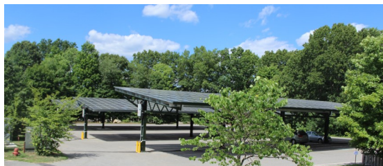
Photo of solar canopy at Congregation Beth Elohim, Acton, MA.
